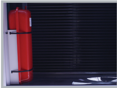
closed expansion tank
